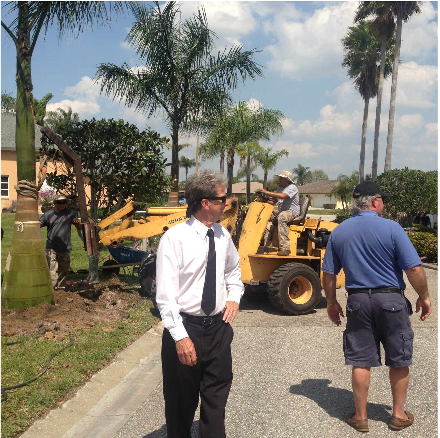
Jim Henry, left, and Rich Delco supervise Vision Horticulture as they install the twelve new Royal Palms along either side of the GVE entrance.
